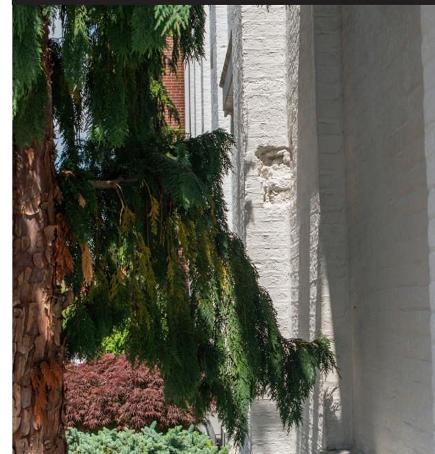
First Presbyterian Church damage sustained from the explosion.
